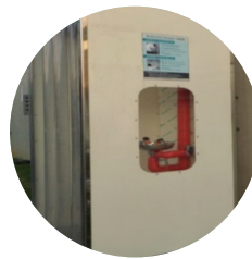
Outdoor emergency washing facility
